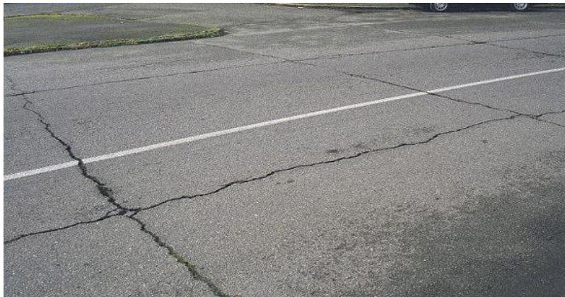
Fig. Joint Reflection Cracks
