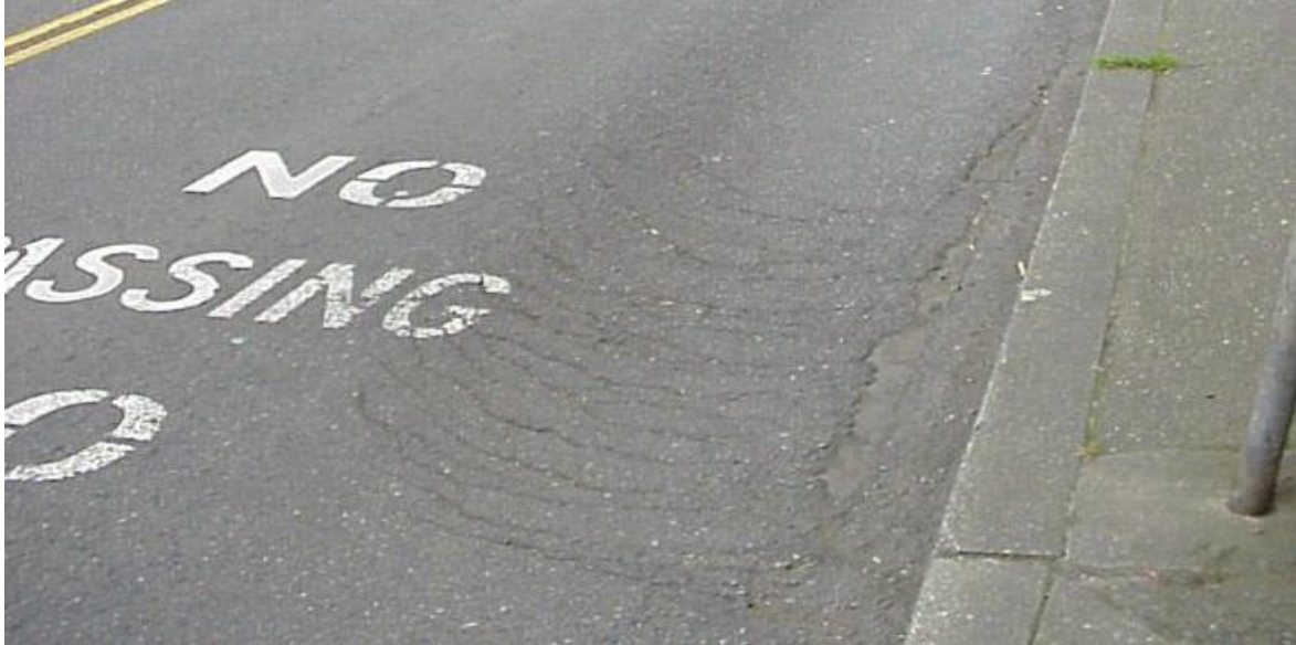
Fig. Slippage Cracks
