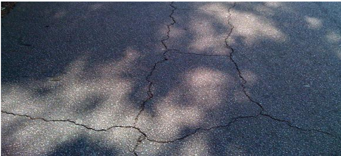
Fig. Block Cracking
